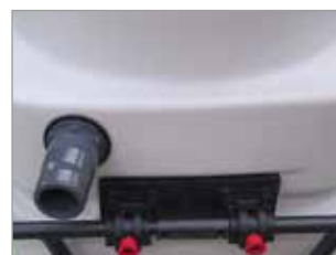
WATER FLOW VALVE
